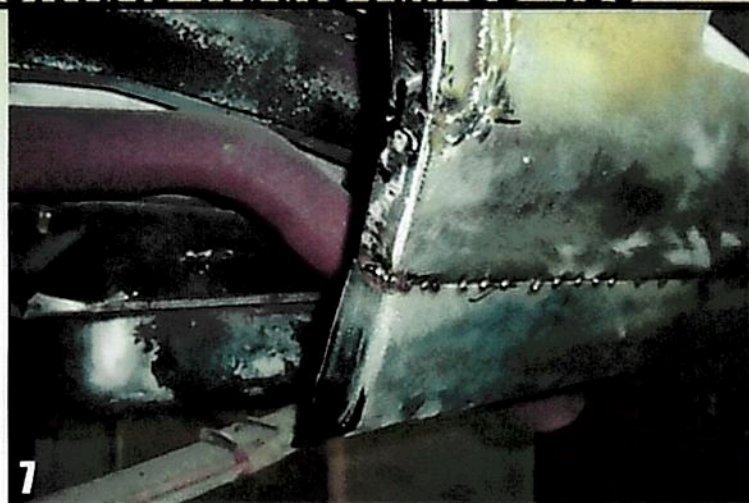
7 The goal was to keep all of the sheetmetal original to the car, so sections were welded in like this repair panel behind the rear wheel.
